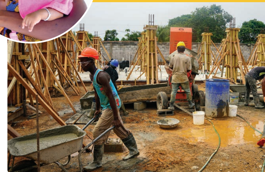
BELOW: Construction crews work hard as the Maternal Center of Excellence buildings take shape. Photo by Sabrina Charles / PIH
